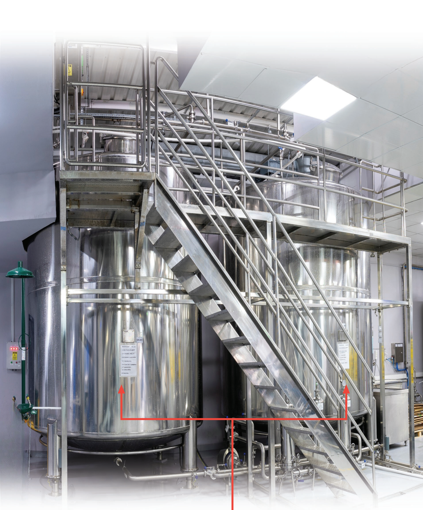
Large Scale Production Tanks 40.000 Liters Capacity
